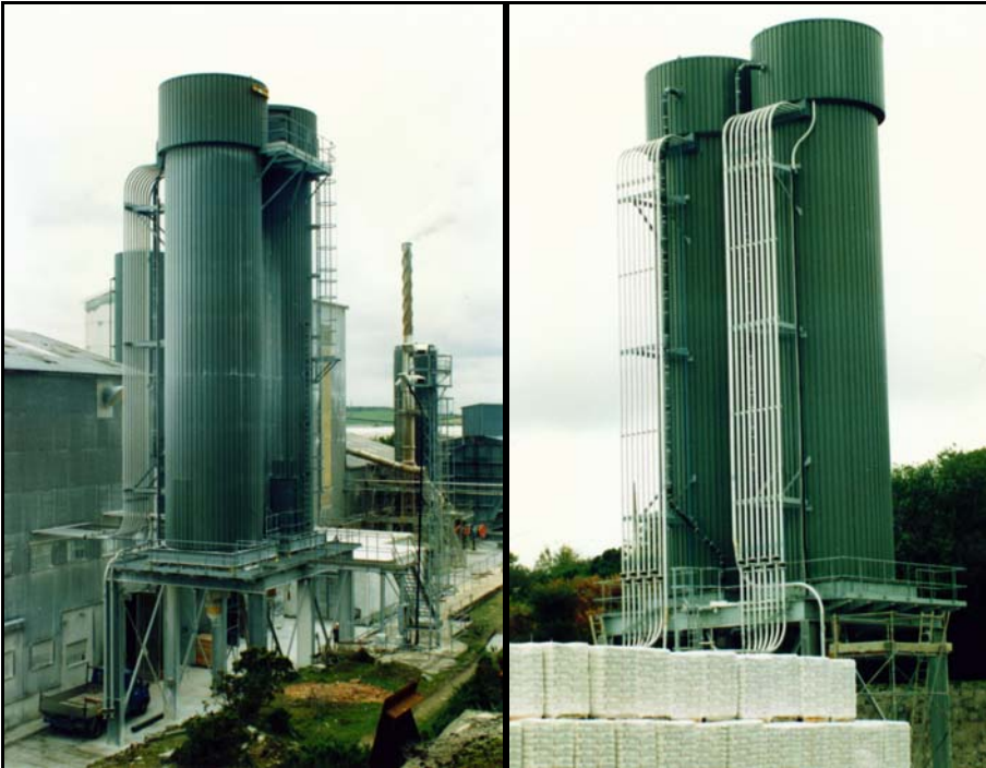
Picture above and below: Lime silos and pneumatic conveying systems installed in Devon and Cornwall.
